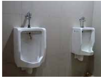
Urinoir flushing system
