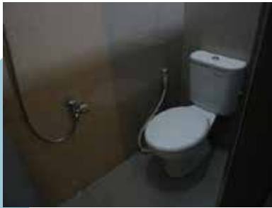
Toilet flushing system
