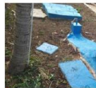
Sistem biogas finished
