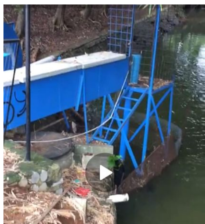
Micro Hydro Power Plant at Salam Lake
