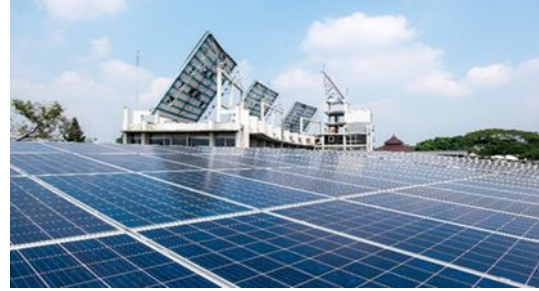
Solar Power Plant of Engineering Center Faculty of Engineering
